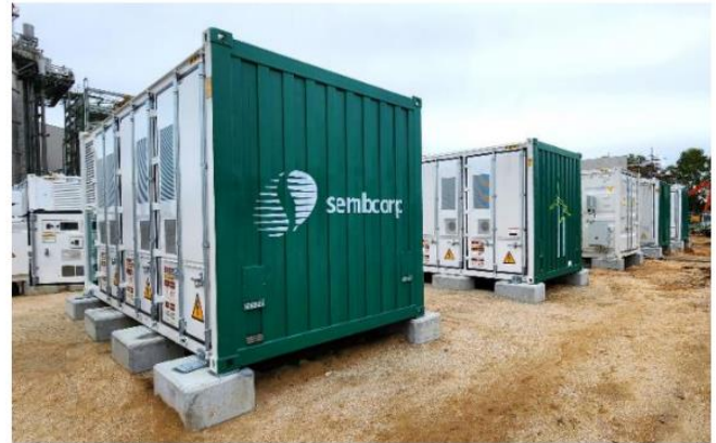
Figure 6: 326MWh Sembcorp ESS is South-East Asia's largest ESS
