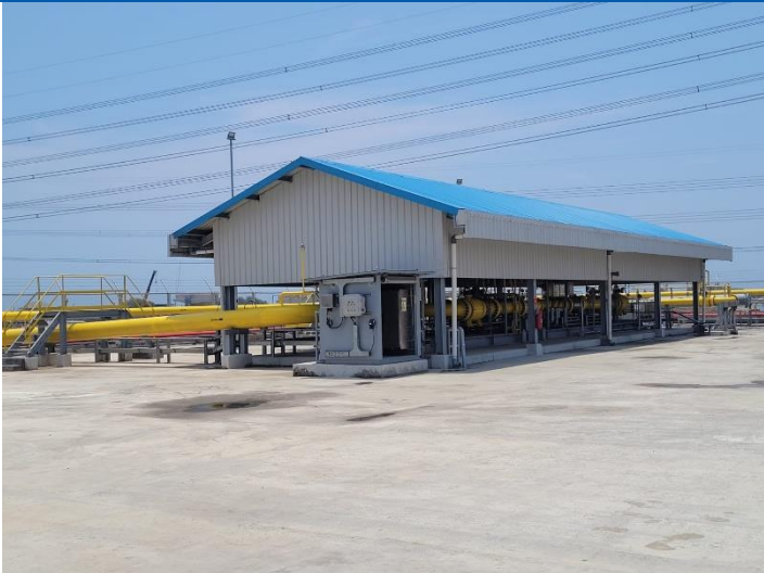
Figure 1: ORF Tambak Rejo facility, Semarang
